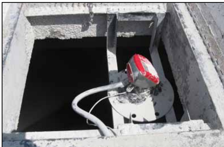
A dusty application in an ethanol plant.
